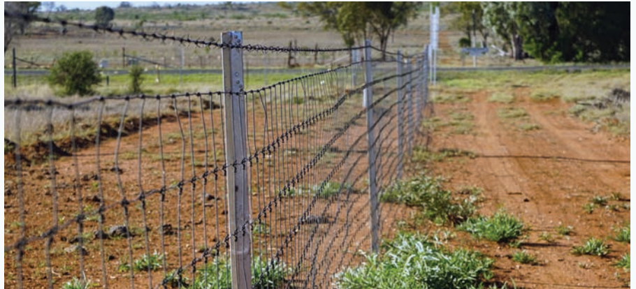
Hitting the wall: Fences will face immense pressure in the months after they have been erected. Maintenance must be kept up as animals learn to respect the barrier. This fence is part of the Morven Cluster and shows evidence of kangaroo impact.
