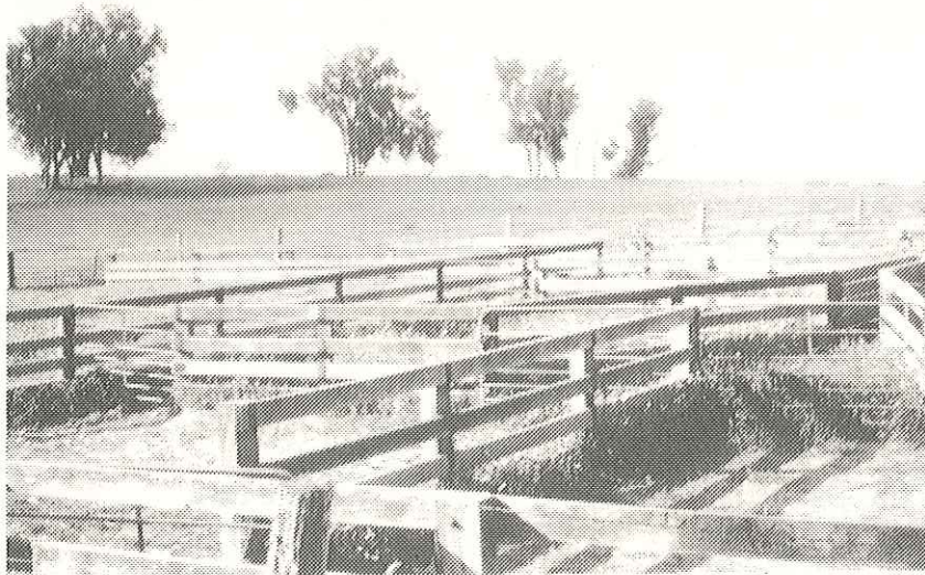
Photo 2. Yards with timber fences. Notice the use of large steel washers on the bolts securing rails to posts.
